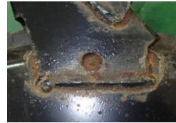
Existing pretreatment (no descaling)
